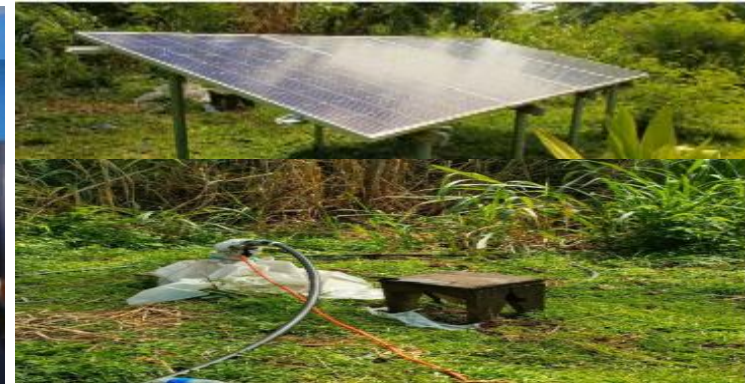
Lelepa Community Borehole
